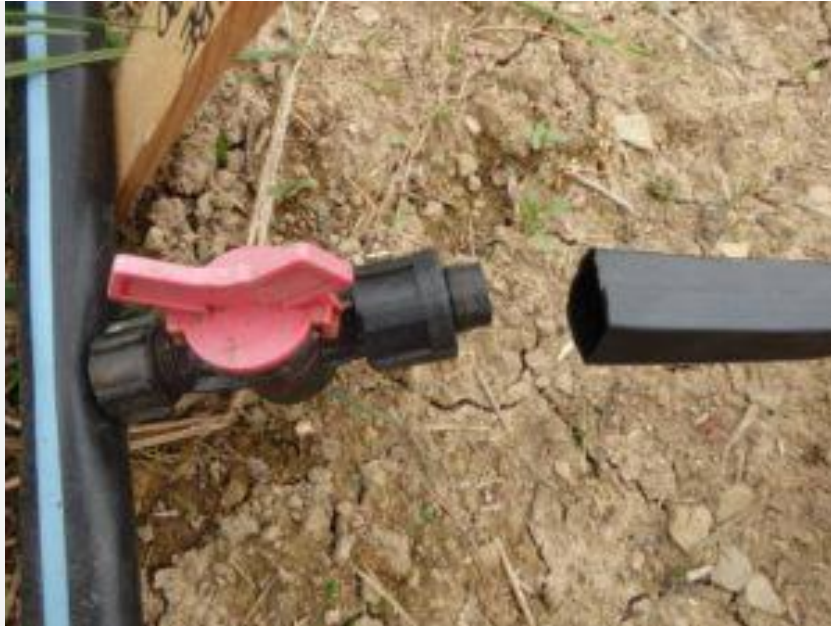
Header Line, Drip Valve, and Drip Tape
